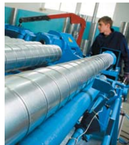
Spiral wound ducts workshop
